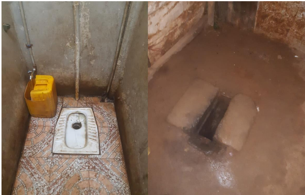
Figure 4.4. Show the common type of toilet and latrine in Juba
