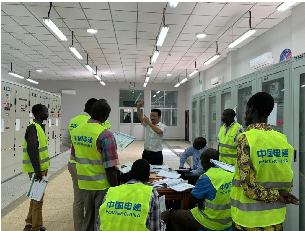
Figure 6.1: Power China staff training local staff in the control room of Ezra Power Plant, Mangala County
